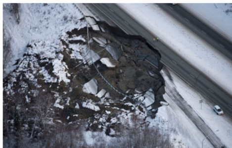
Figure 1. Failure of Glenn Highway embankment induced by the 2018 Anchorage Earthquake 2 .
